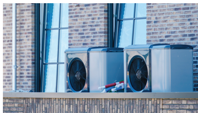
Air source heat pumps installed in an urban setting. Photo: Shutterstock
